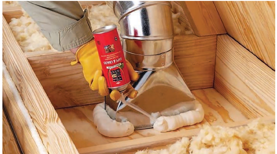
Providing a continuous, generous, and reliable air seal around every penetration in the attic floor is becoming increasingly critical for code compliance and indoor health.
